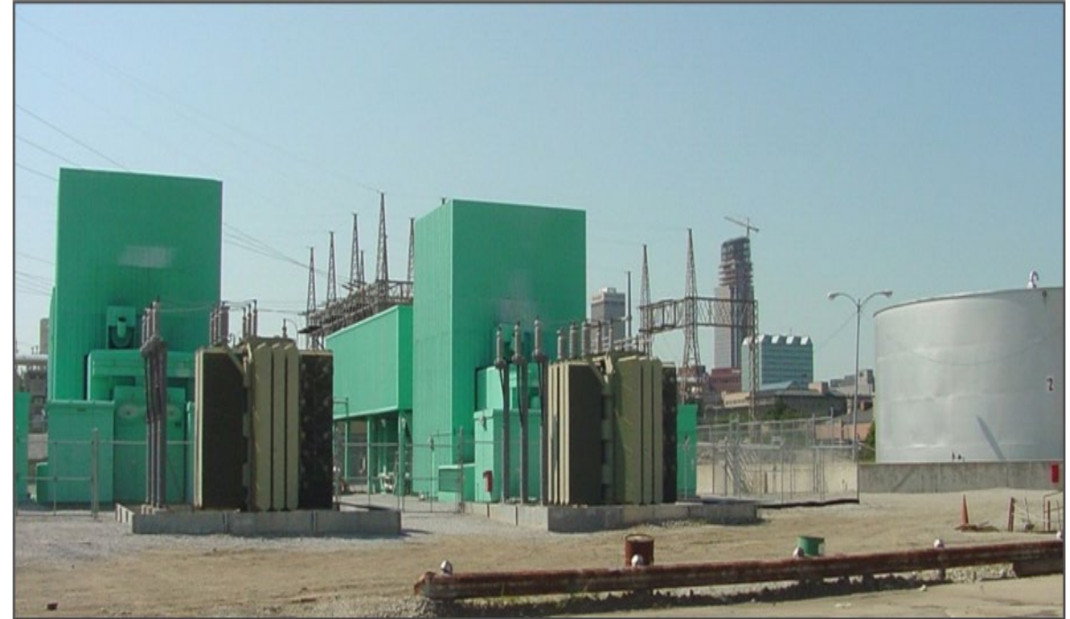
Omaha Public Power District Jones Street Station 1 & 2
