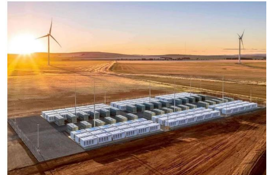
The Hornsdale Power Reserve is located approximately 16km north of Jamestown in South Australia.
