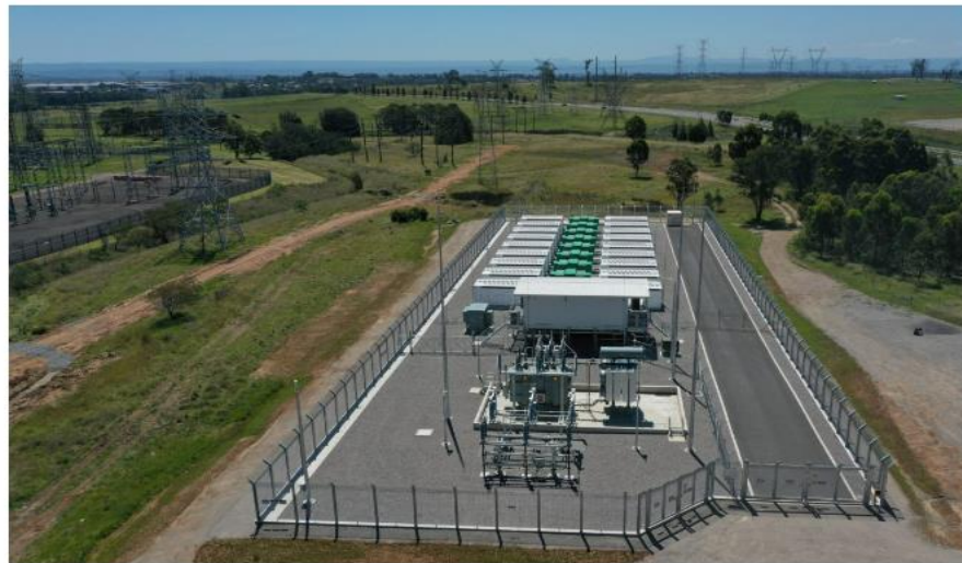
The 50 MW/75 MWh Wallgrove Grid Battery is now fully operational.
