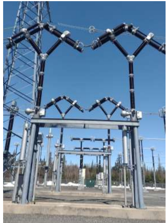
Figure 1: The Failed Air Blast Breaker
