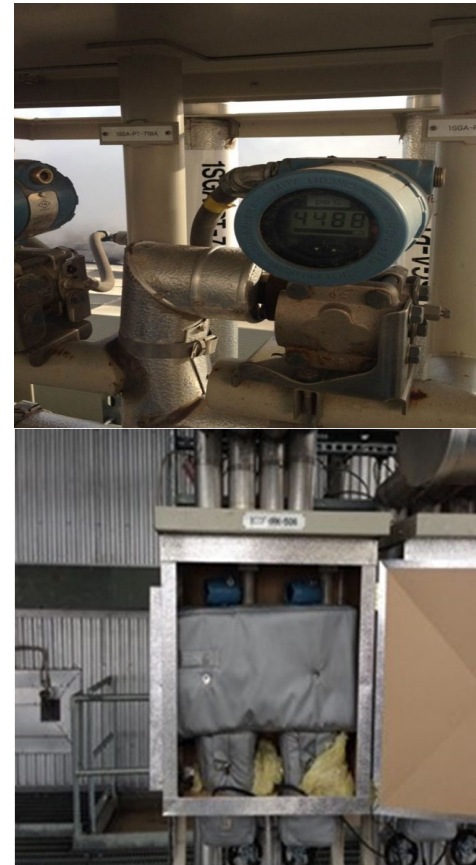
Relocated transmitters – protected from elements
