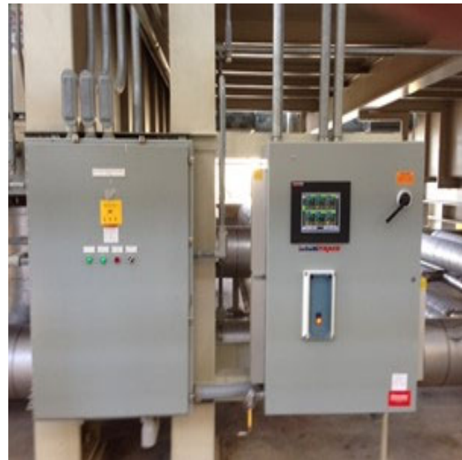
Older style heat trace panel
