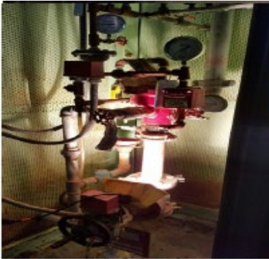
Lube Oil Building GT1/2
