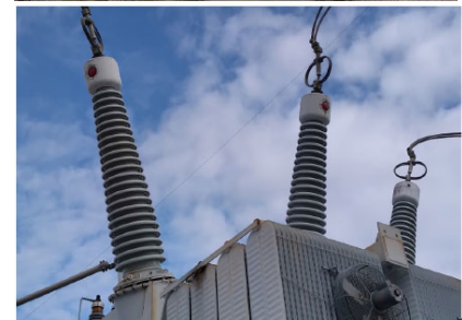
Transformer Bushing Oil Level
