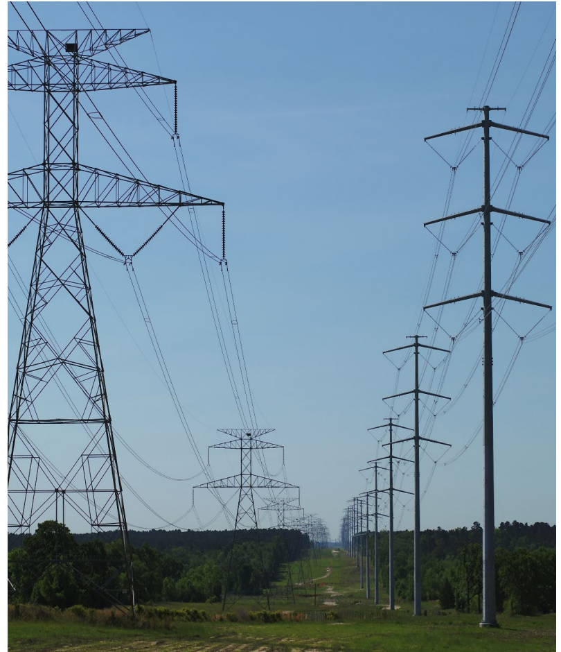
Brazos Valley Connection image courtesy of CenterPoint Energy
