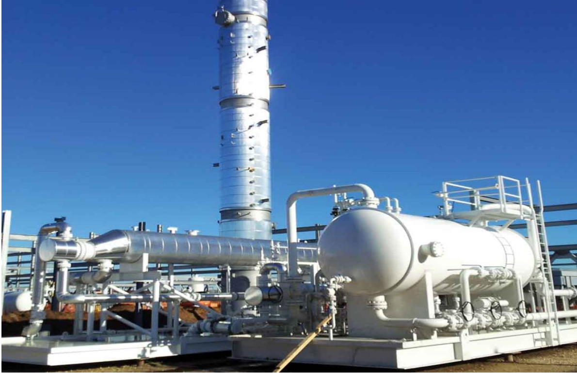
Figure 4-12 Stabilization unit (Source: Schlumberger)
