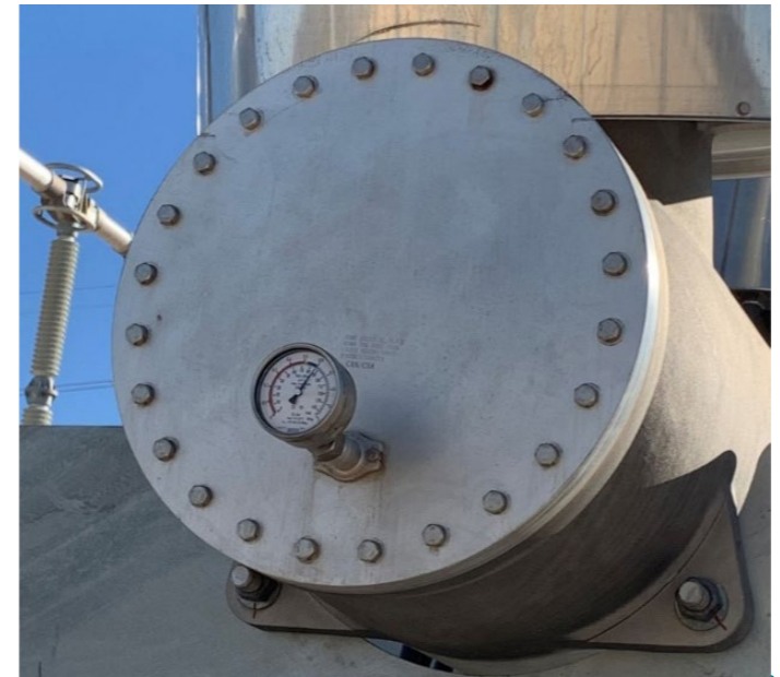
Local Pressure Gauge on SF6 Insulated Breaker
