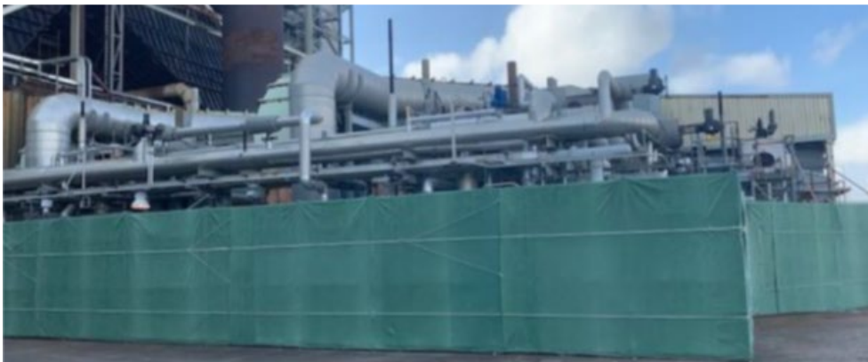
Temporary Wind Break Structures
