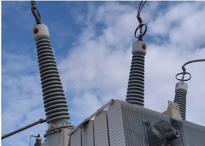
Transformer Bushing Oil Level
