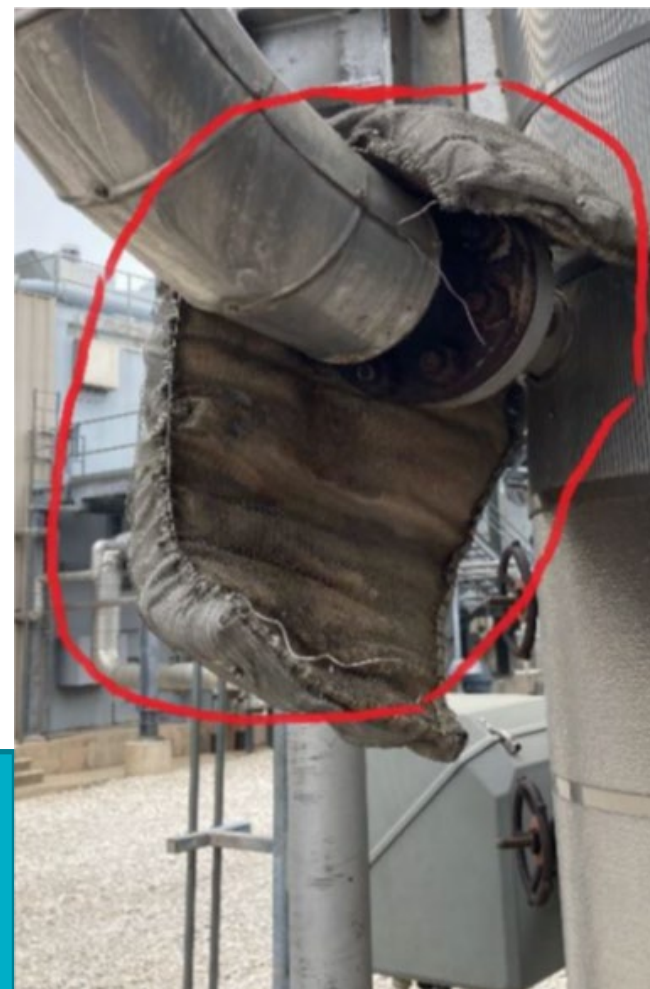
Incomplete Insulation Blanket above, "Clamshell" Instrument Enclosure below
