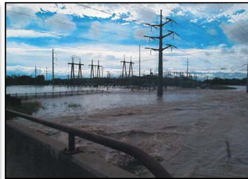
Ben Davis Substation during 2015 Flood
