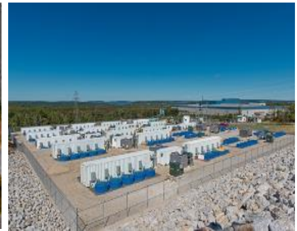
Hazle, PA 20 MW Facility Initial COD Sep 2013 Full COD June 2014
