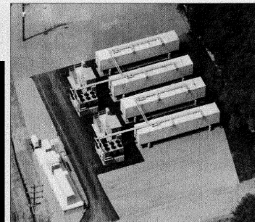
Energy storage facility in Johnson City, N.Y.
