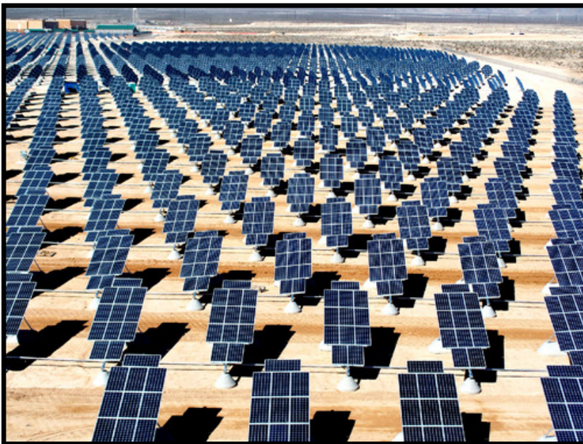
Photovoltaic Array (15 MW) – Nellis Air Force Base, Las Vegas, NV
