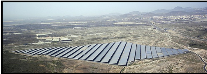
SOLTEN II (11 MW) – Granadilla Industrial Estate, Canary Islands
