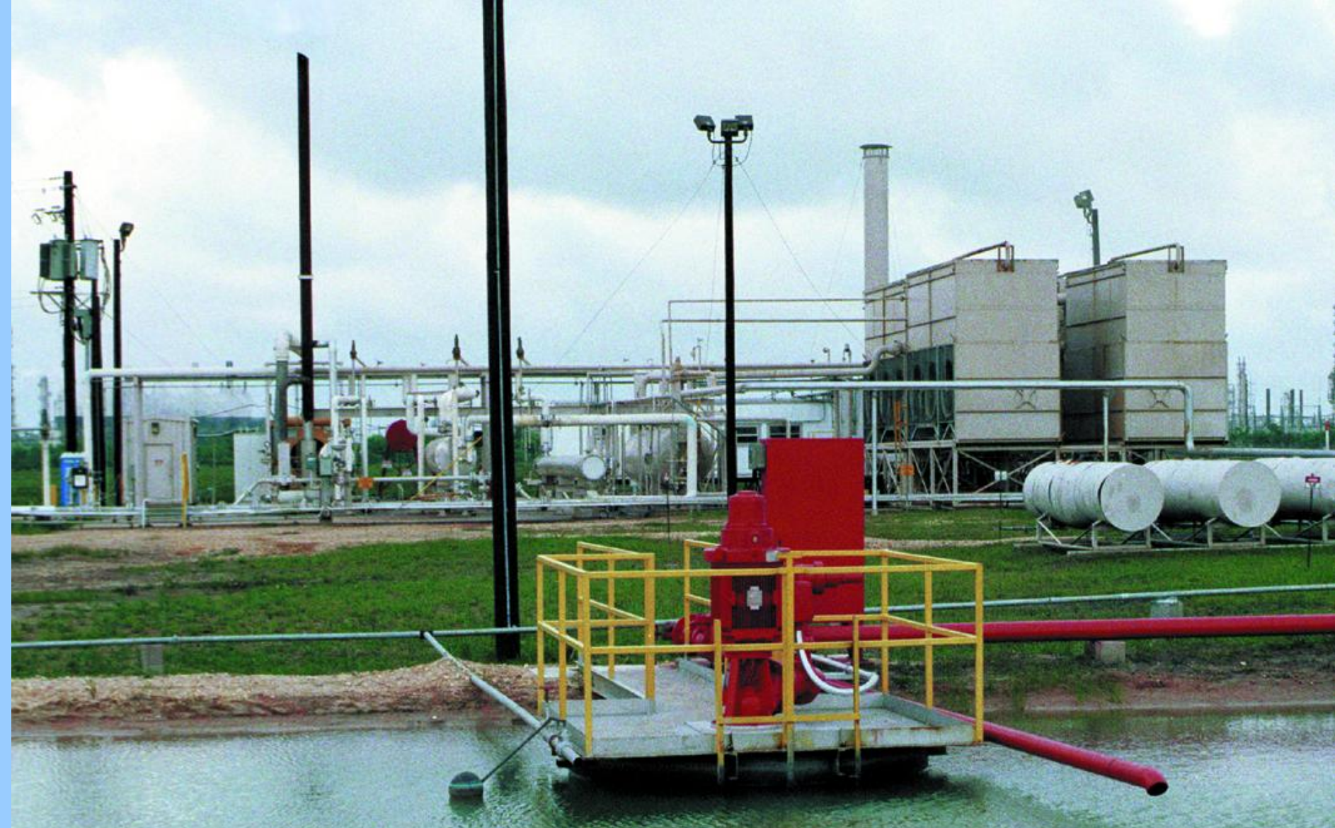
Pleasant Bayou, Brazoria County Texas Power Plant USDOE Geothermal Project, ½ gas ½ Geothermal 1 MW produced between mid 1989 and mid 1990,
